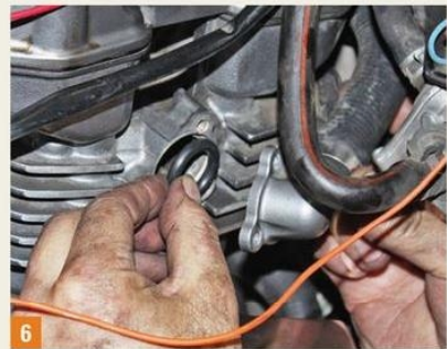
6 With the hoses prepared, you can simply reinstall the parts. Here a new O-ring is fitted to be sure of a leak-free connection.
